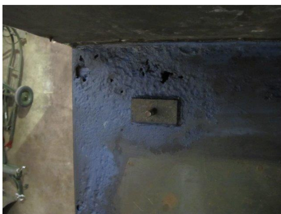
Corrosion in the mild steel sheet – pedestal roof section
