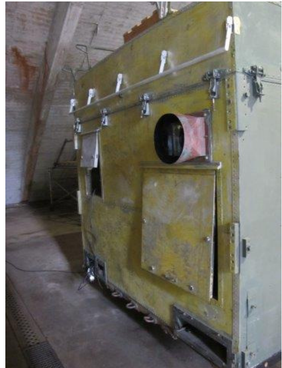
End wall of LCP cabin
