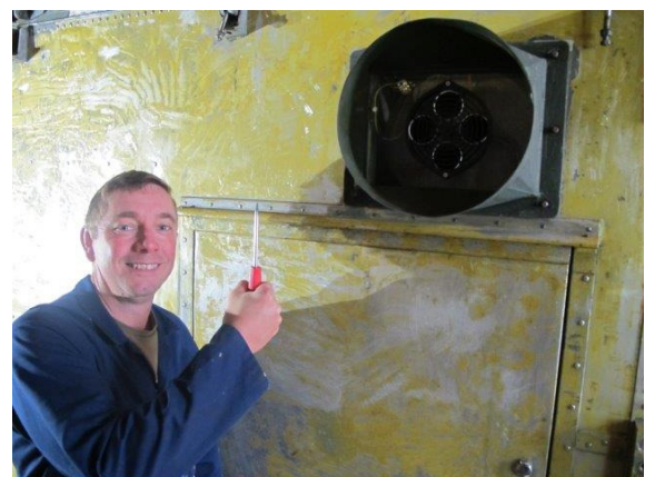
New LCP Extractor Fan I made it (the fitting not the fan) – Pete Murray
